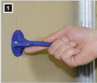
1 Adhesion of the bus holder on the reverse side of the first cladding
