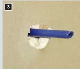
3 The dry wall constructor hammers a hole and lets the central spine protrude; this serves for centring the drill bit.
